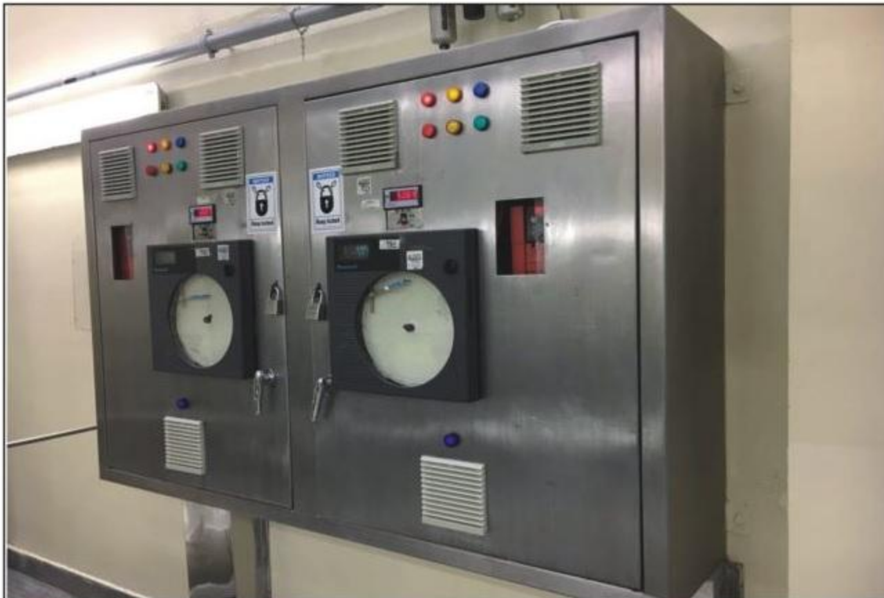
Control Panel for Steam Jacketed Vessel
