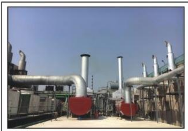
5.25 TPH @ 10 Bar (G) Each Waste Heat Recovery Boiler
